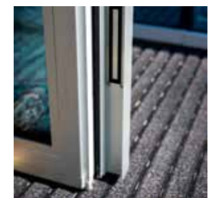
Concealed electromagnetic lock on the opening frame
